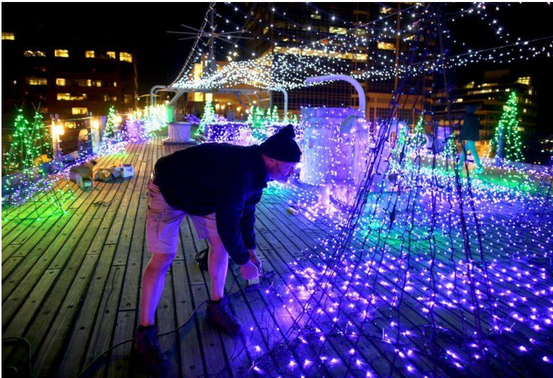
Jeremy Kilgore, owner of Blue Steel Lighting, continues setting up lights on the deck of the USS Wisconsin on Monday, Nov. 16, 2020, for the upcoming WinterFest on the Wisconsin.
